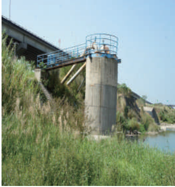
River Water Intake Well
