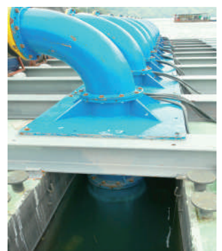
Raw Water Intake
